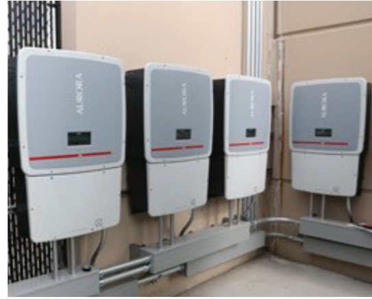
Today's solar inverters convert DC to AC power, but do not provide adequate Reactive Power.
